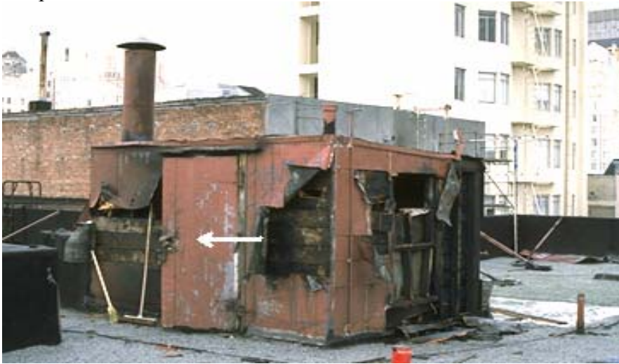
Penthouse door which was forced open during a fire in a Tenderloin SRO.
